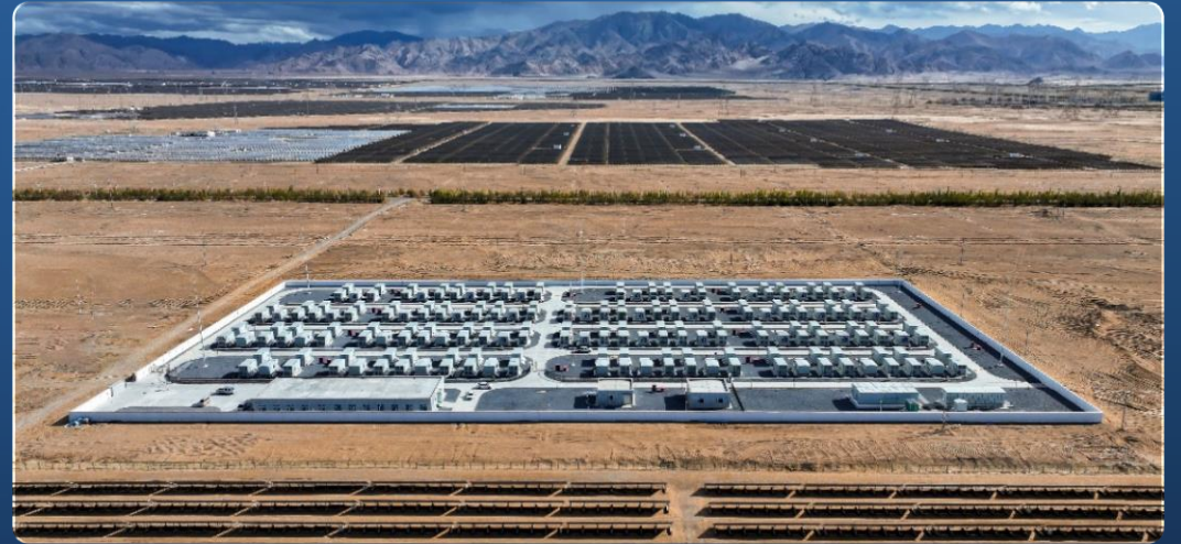
📍 Qinghai, China Geermu Shared Energy Storage Station Project
